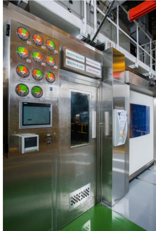
Facility Local Operator Panel
