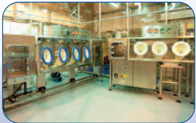
Isolators in Test Area
